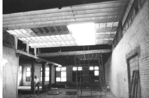
1992 | About one-third of the roof structure was removed and reframed to form the upstairs entry hall light monitor. The windows were replaced with modern insulated glass units matching the historic double-hung and transom units.
