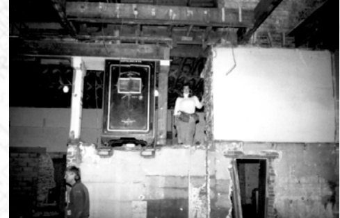
1992 | The Barteldes Seed Company safe was left suspended atop a brick wall after the old mezzanine was demolished. This antique Diebold safe from the early 1970s weighs two tons and was hoisted onto new floor beams above.
